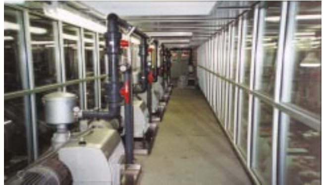
Vacuum pumps in glass enclosure
